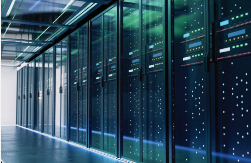
Server room. Source: Getty Images
